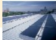
Solar cooling installation using DDC technology and air collectors in Central Europe (Source : Fraunhofer ISE)
