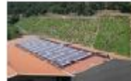
Solar cooling installation for a wine cellar in South of France (Source : TECSOL)
